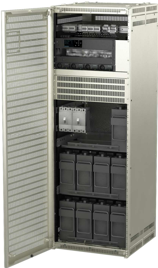
IBB SYSTEM IN FPC CABINET
