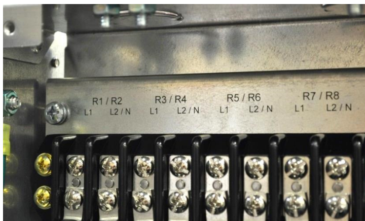
Figure 31 – Barrier Strip Terminals
