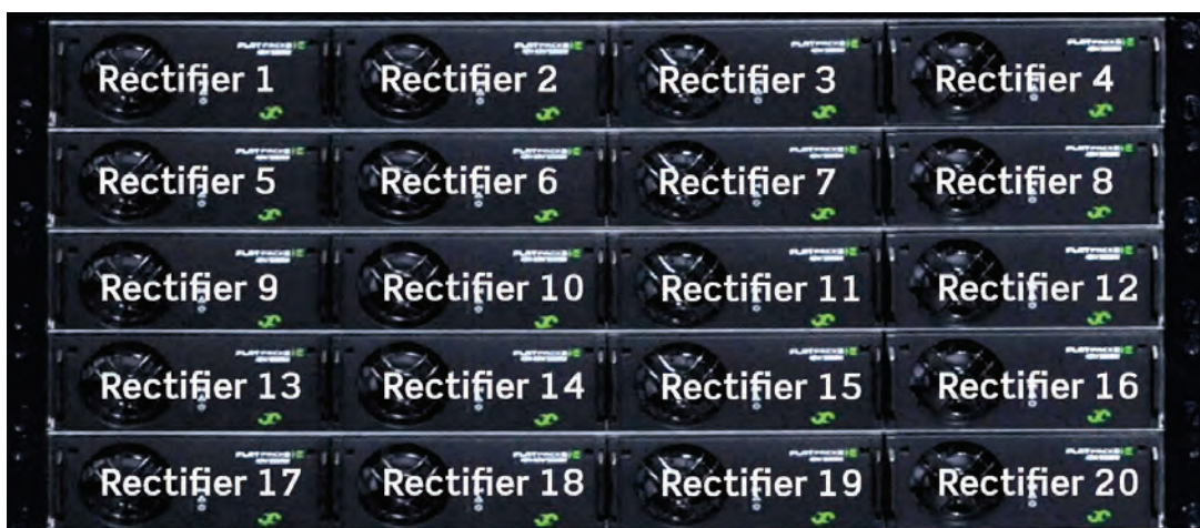
Figure 7 - Rectifier Slots (numerical order)
