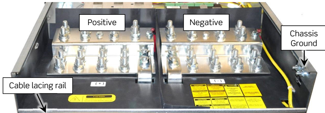
Figure 17 – Bulk Load Connections
